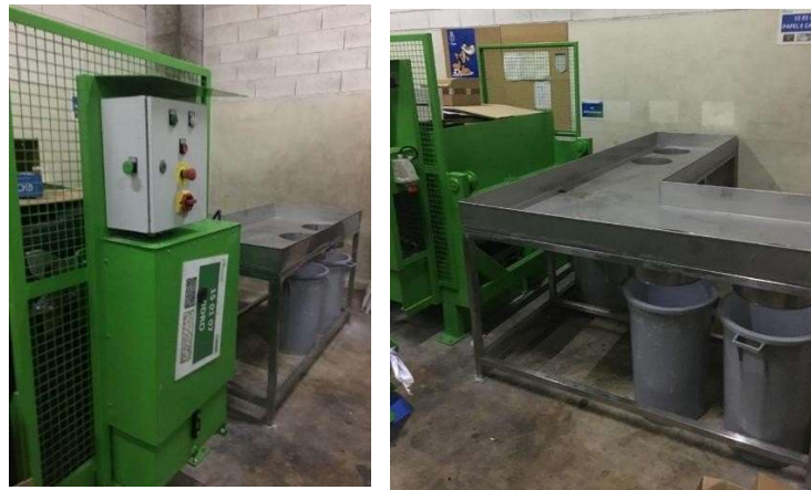
Figure 13. The installed sorting station
